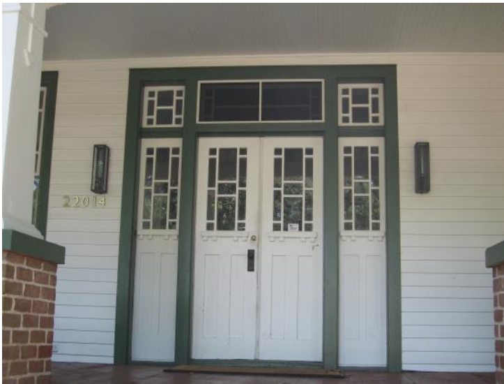
This entrance has its original multi-light double doors, sidelights, and transom (22014 2nd Street).
