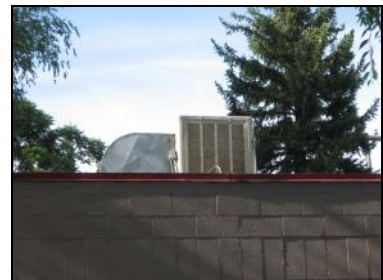
Example of a roof mechanical system which is set back from the street and not readily visible.
