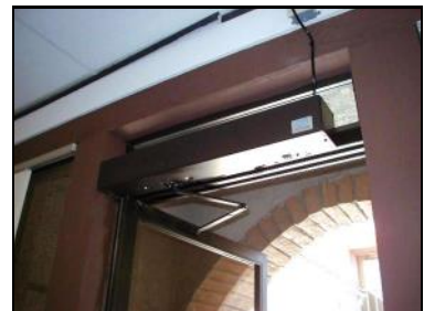
Doors can also be modified with pressurized door openers to allow for ease of access.
