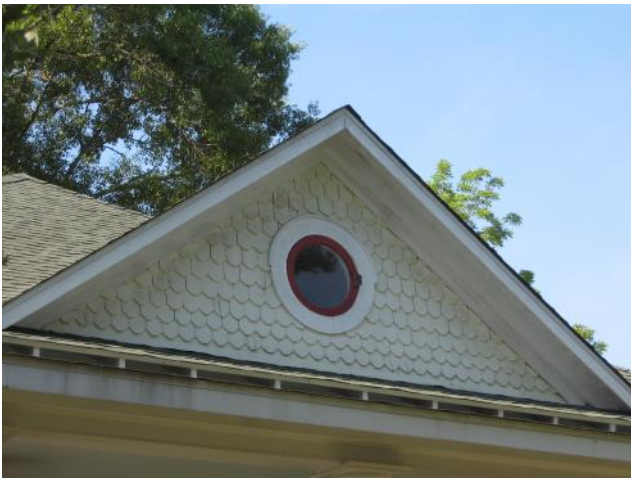
Left: Original wood shingles in the gable field at 22200 Main Street.
