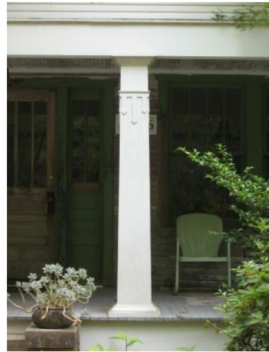
When wooden elements like porch columns require repair or replacement, they should be rebuilt to match their original design or in a style compatible with the style of the dwelling. This Bungalow style column was rebuilt after being damaged by Hurricane Katrina (71446 St. Joseph Street).
