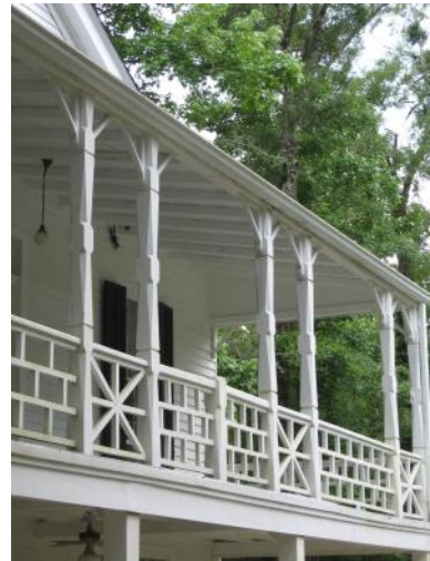
Porches such as at 22128 5th Street have an abundance of wood elements, including milled posts, railing and balusters, and ornamental trim.
