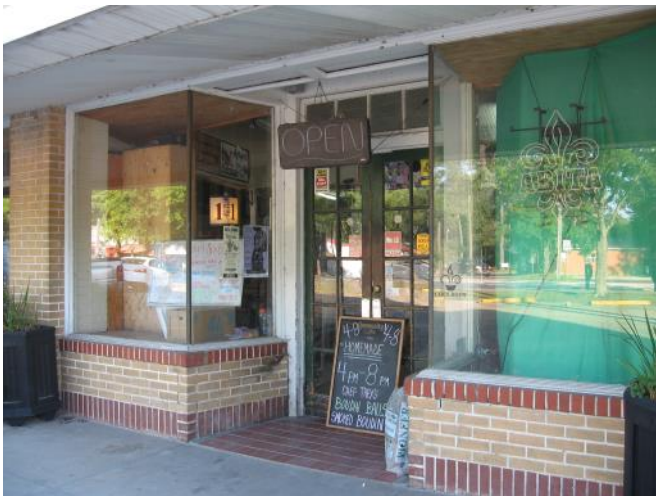
The 1903 Rauch's Grocery (Abita Springs Market) original storefront has a recessed entrance flanked by display windows on brick bulkheads (22069 Highway 59).
