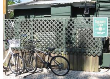
Lattice panels are used to screen the HVAC units at 22132 Level Street.
