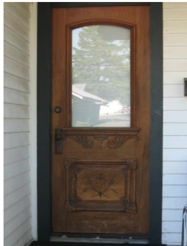
Decorative wood and glass doors as at 72050 Hickory Street should be maintained and preserved..
