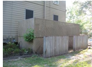
Appropriate screening of HVAC units at 22070 Highway 59.
