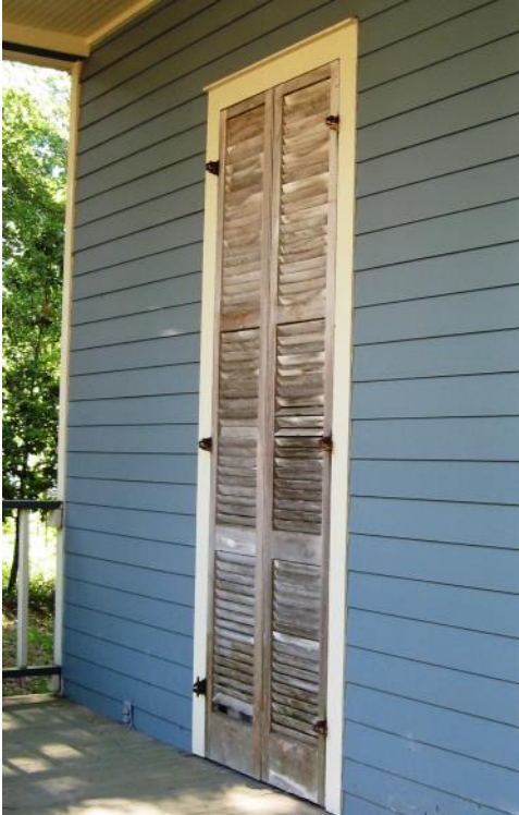
Original window shutters protect the window behind them and these shall be preserved and maintained.
