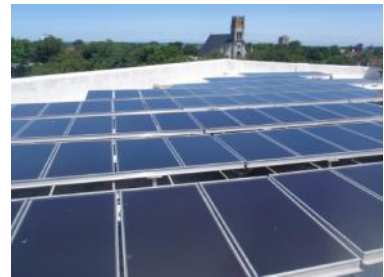
Example of appropriately mounted rooftop solar panels on a commercial building.
