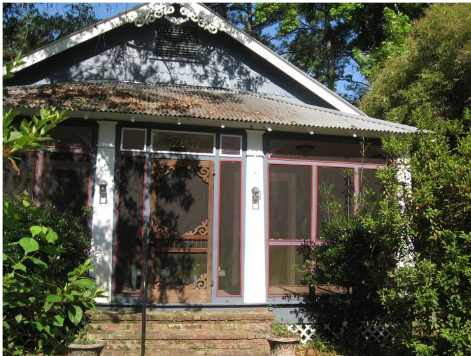
This porch at 72037 Laurel Street is appropriately screened, with sections inserted within the openings between its columns.
