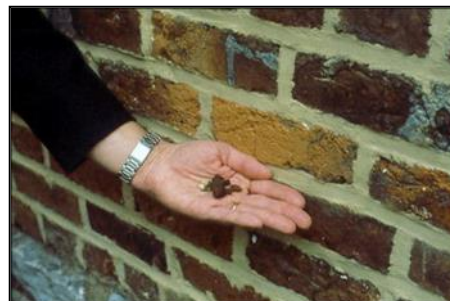
No—Do not use any abrasive cleaning on historic brick walls which could lead to spalling and cracking.
