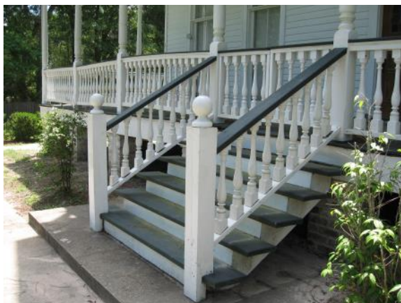
Wood porch elements and stairs should be preserved and maintained (71648 Maple Street).
